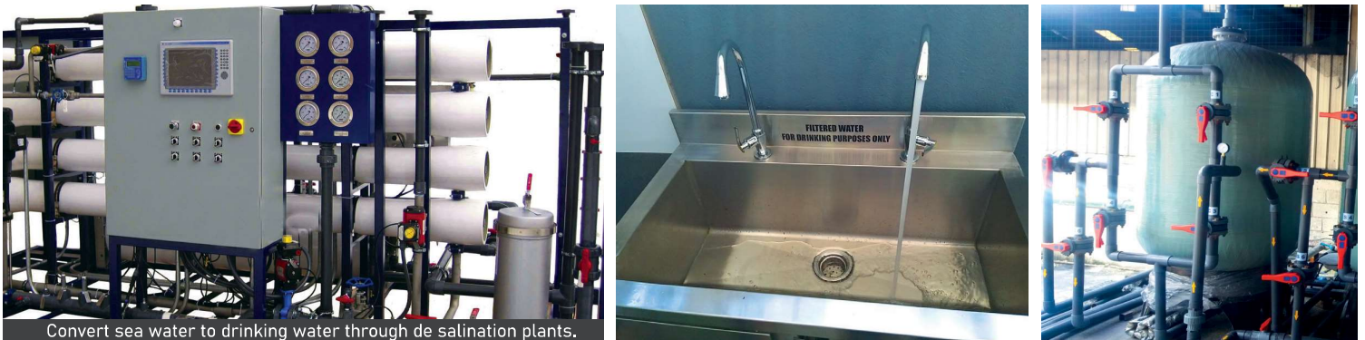
Convert sea water to drinking water through de salination plants.
